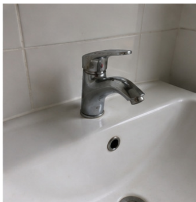
Sanitary fitting evidence
